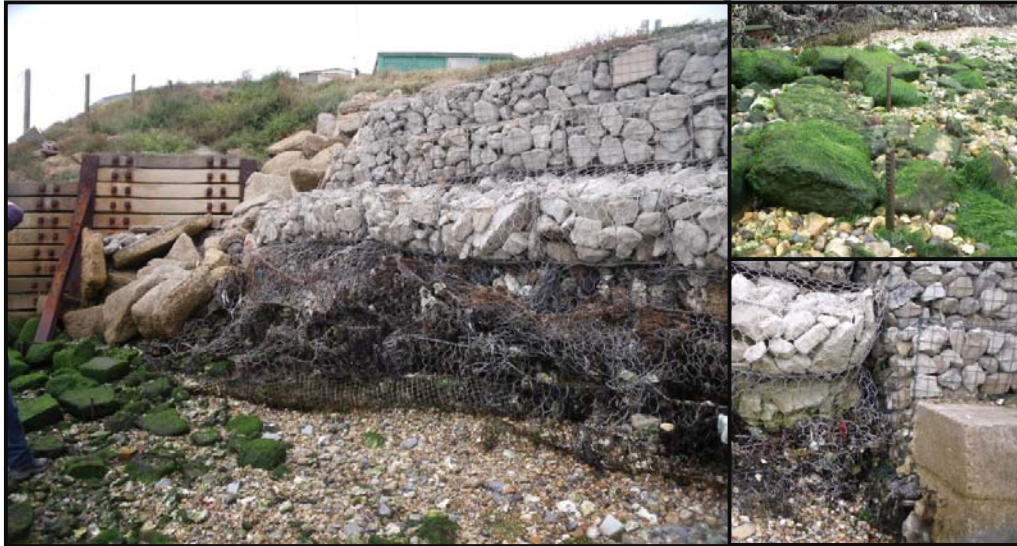
Figure 6: general arrangement of Defence Length 5, including images of protruding bars and broken gabions
