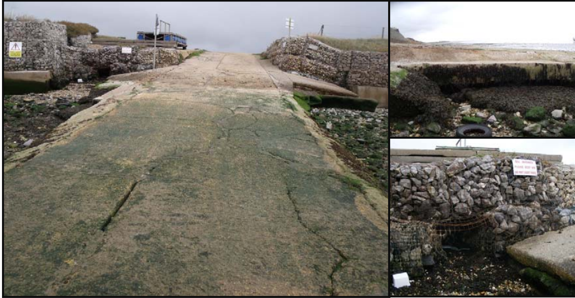
Figure 5: general arrangement of Defence Length 3, including detailed images of undercutting and gabion damage
