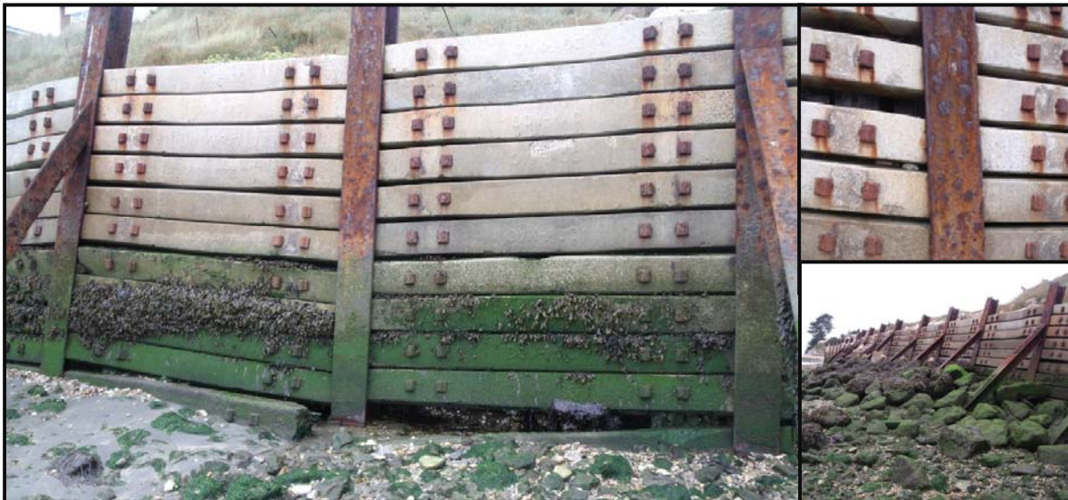
Figure 7: general arrangement of Defence Length 6, including images of corrosion and rock armoured toe
