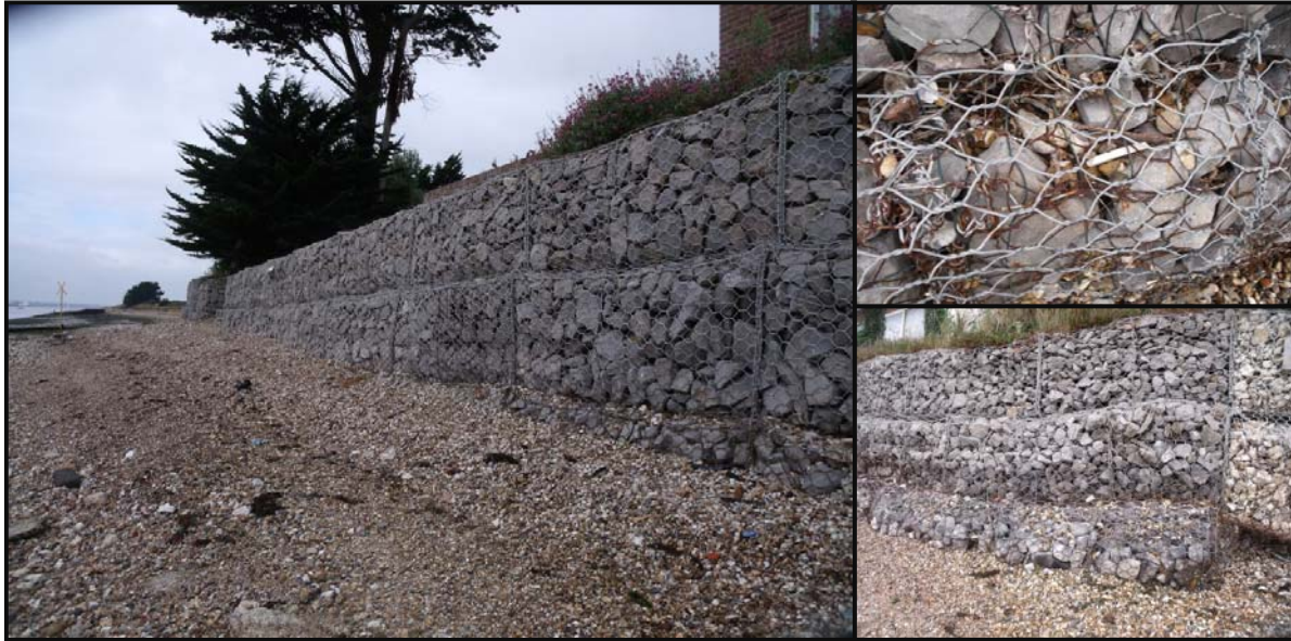
Figure 10: general arrangement of Defence Length 9, including detailed images of mass concrete pours and gabions
