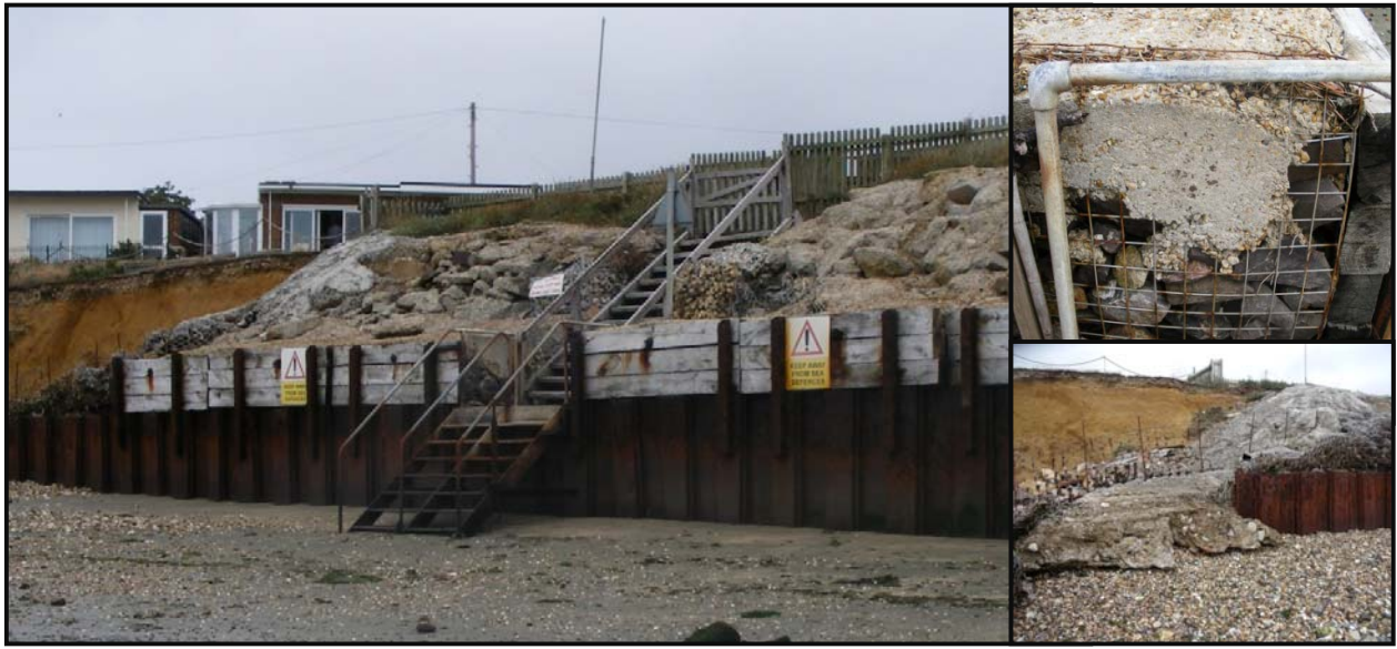
Figure 8: general arrangement of Defence Length 7, including images of mass concrete pours and gabions
