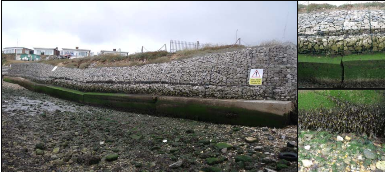
Figure 5: general arrangement of Defence Length 4, including detailed images of undercutting and large toe wall cracks
