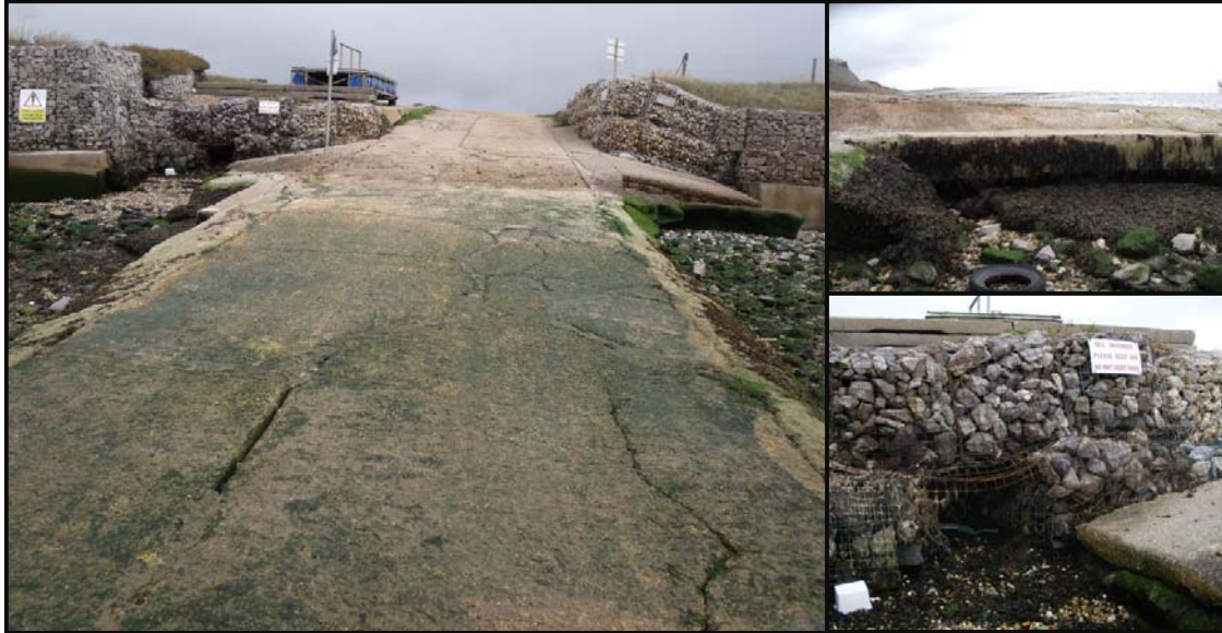
Figure 5: general arrangement of Defence Length 3, including detailed images of undercutting and gabion damage
