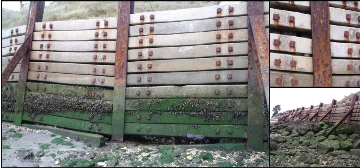
Figure 7: general arrangement of Defence Length 6, including images of corrosion and rock armoured toe
