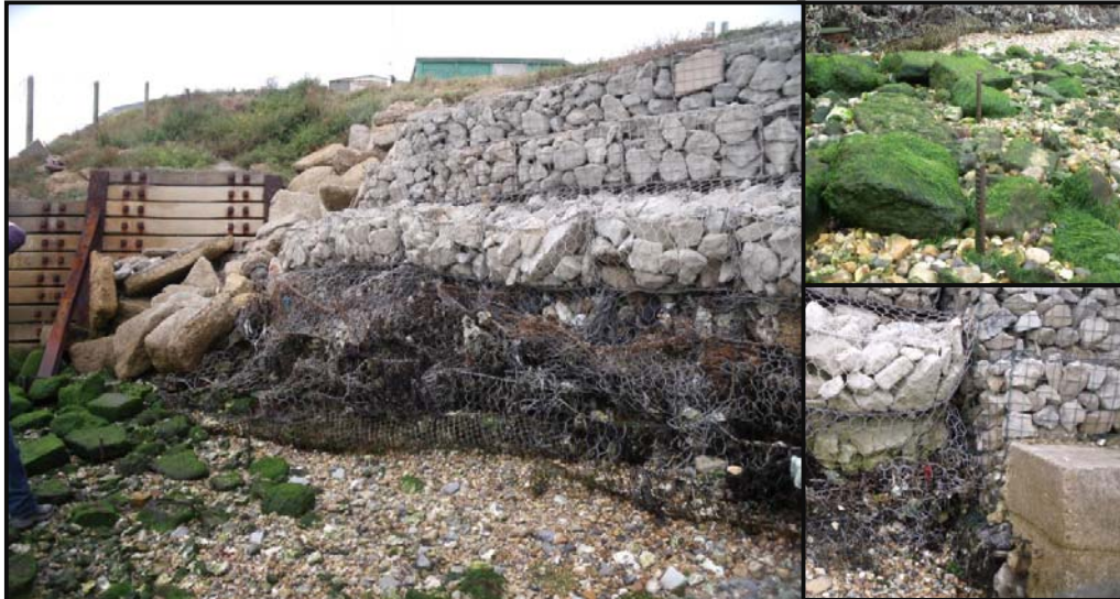
Figure 6: general arrangement of Defence Length 5, including images of protruding bars and broken gabions
