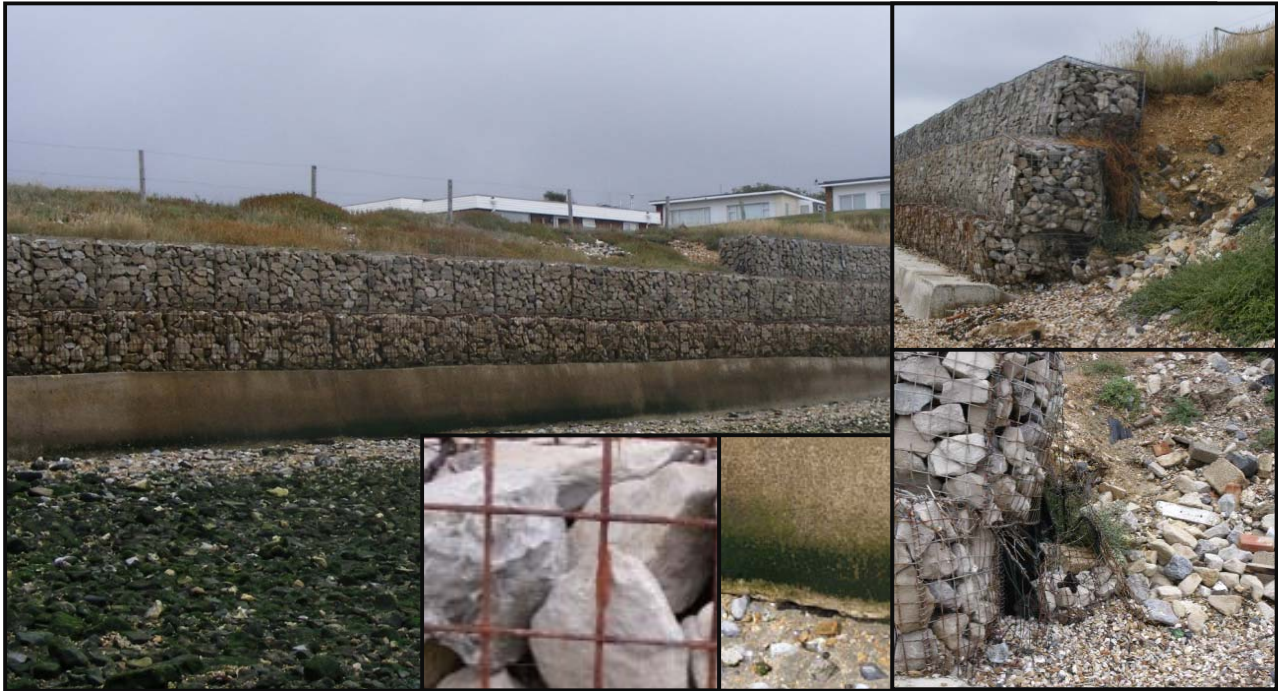
Figure.4: general arrangement of Defence Length 2, including detailed images of undercutting, damage and corrosion
